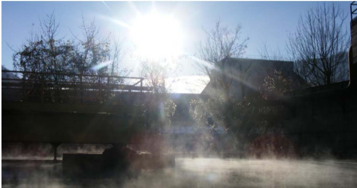
Wastewater treatment plant and fume aspiration system
