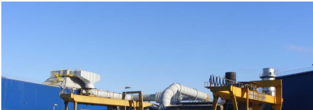
Fume suction and filtering system realized in 2010
