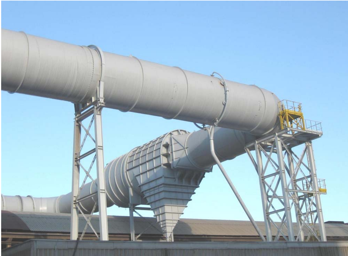
Fume suction and filtering system realized in 2010
